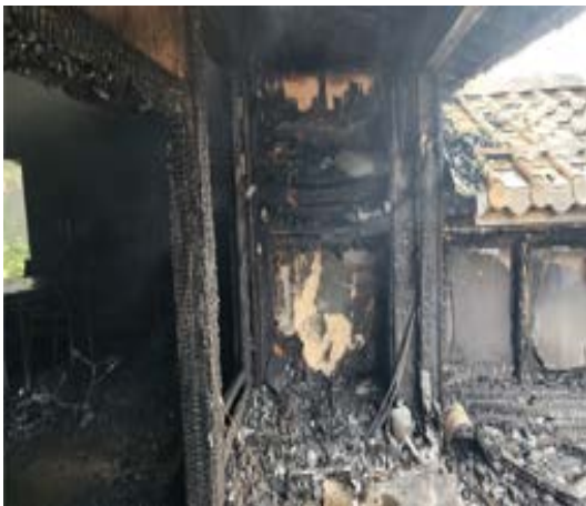
Fig. 3 a photograph of the burning of a wooden building
