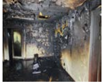
Fig. 7 House Living Room Burn Photo 1
