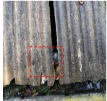
Fig. 6 Fire origin point
