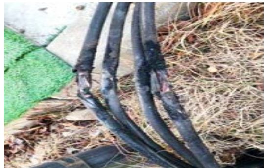
b. Insulation-failed wire
