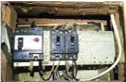
a. Deteriorated electrical equipment
