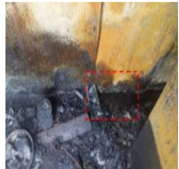
Fig. 9 Fire origin point
