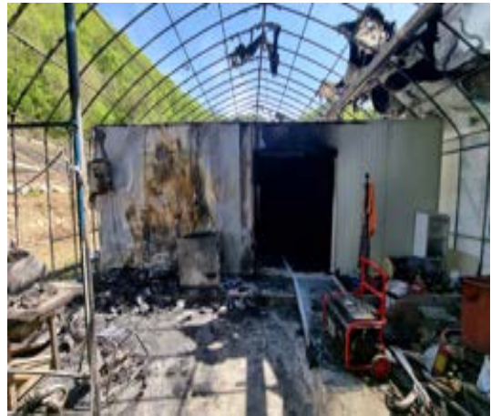
Fig. 2 Burn photo outside the building
