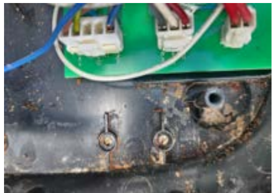
Fig. 12 Water stains observed beneath the PCA board
