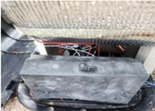
Fig. 9 Protective cover for PCA and wiring
