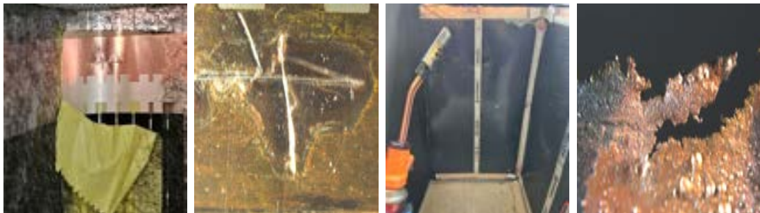
Fig. 26 Damage to copper foil bus bar
