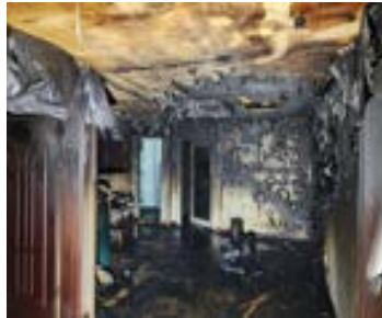
Fig. 9 House Living Room Burn Photo 3
